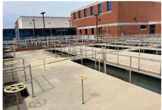
Filter Sedimentation Basin Drain and Influent Valves
