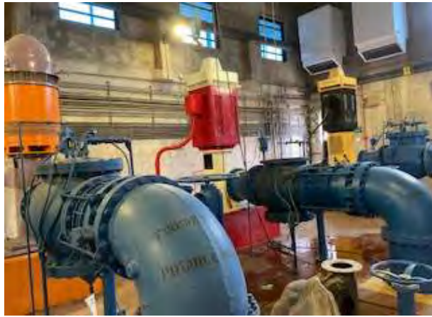
High service distribution pumping equipment
