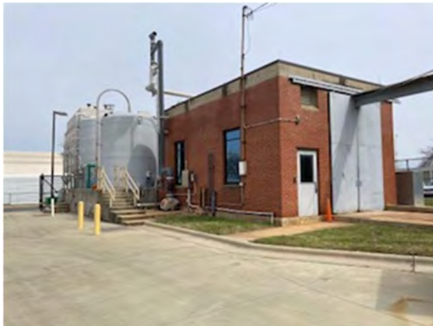
Sodium Hypochlorite On-site Generation System
