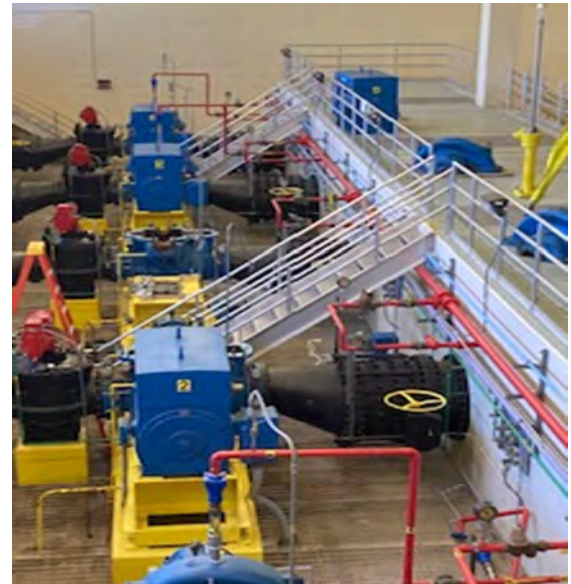
Raw water pumping equipment
