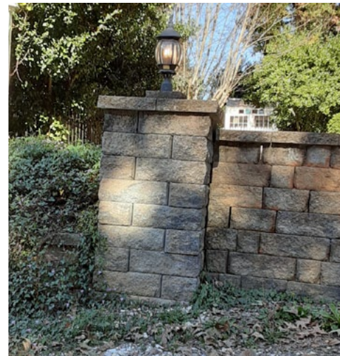
Decorative lighting fixture on masonry column
